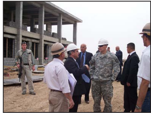
The author inspects the on-going construction of a Police Academy in Irbil, Iraq.
