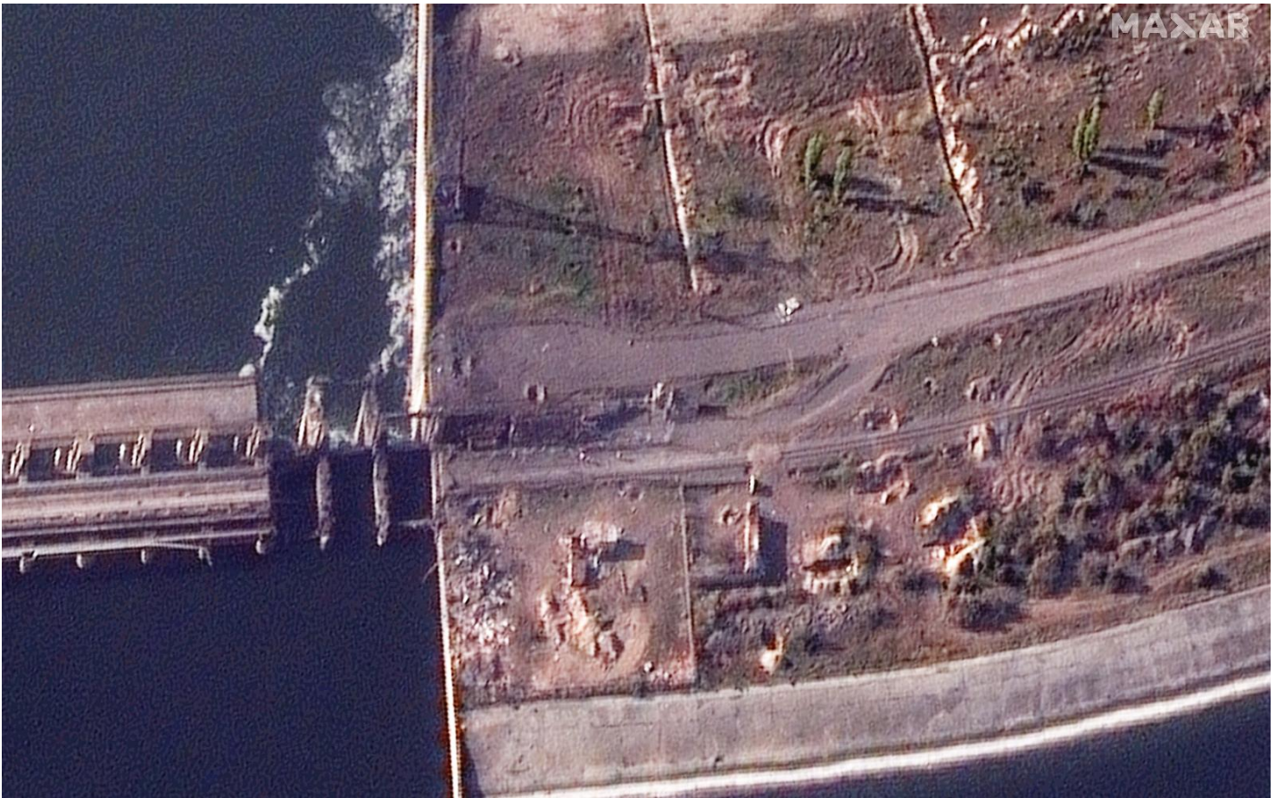
Closer view of damage to the damaged section of the Nova Kakhovka dam on November 11. Source: Satellite image ©2022 Maxar Technologies
