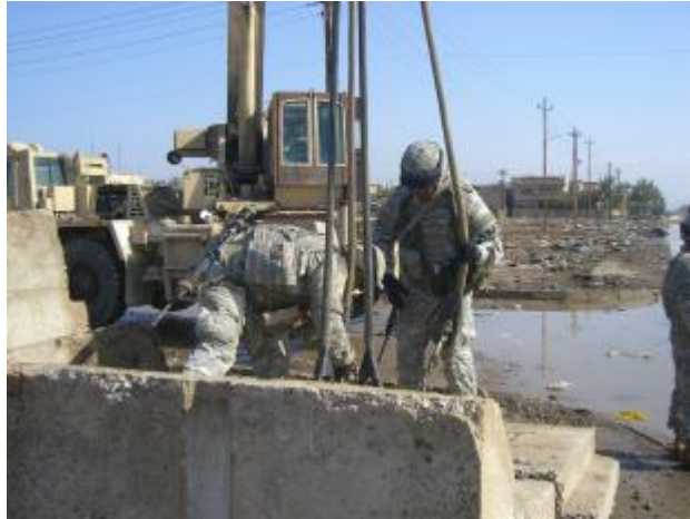
Soldiers from 887th Engineer Company secure a concrete barrier for movement into place around the perimeter of a new combat outpost in the Ghazaliya neighborhood of Baghdad. (U.S. Army photo by Capt. David Hudson)
